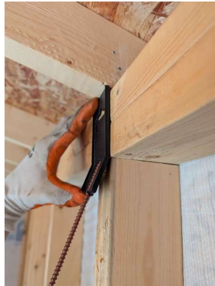
Figure 2. Placement of 6" truss screw in angle guide to ensure proper installation angle
